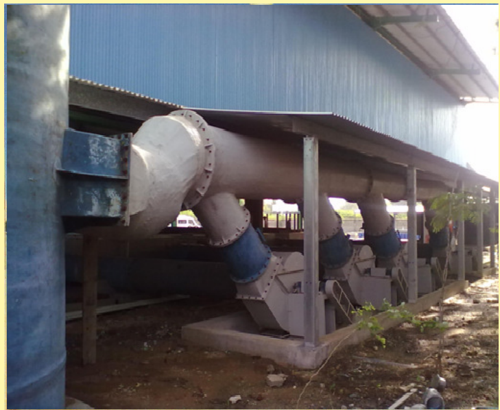
SCRUBBERS FOR ACID FUMES
